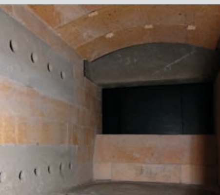
Fully fireclay lined combustion chamber.
