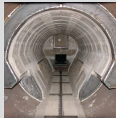
Combustion chamber with de-ashing chain.
